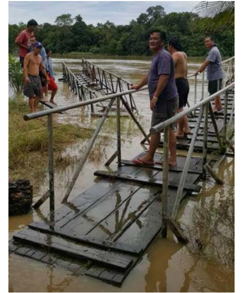
Jetty and pontoon damaged by flooding. Malaysia. Photo courtesy of SAVE Rivers Network
